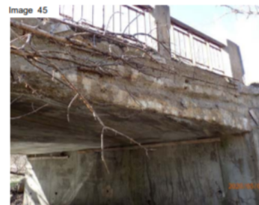
NW fascia major disintegration
