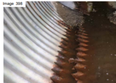
Mid east wall fill leaking
