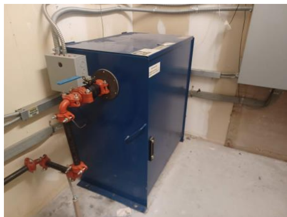
Photo 12: View of the hydraulic unit for the passenger elevator for the second floor commercial units at 1105 D Kingston Road.
