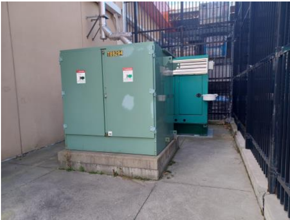
Photo 7: View of the transformer and diesel powered generator located east of the Site building occupied by Home Depot. Photograph taken facing west.
