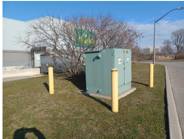
Photo 8: View of the transformer observed to the south of Food Basics. Photograph taken facing east.
