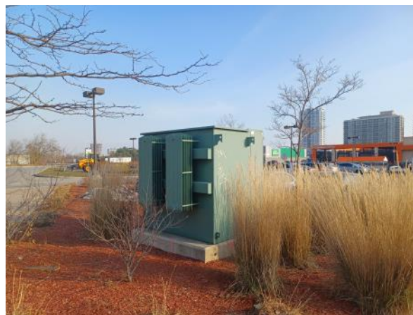
Photo 10: View of the transformer located between the water building and 1105 E Kingston Road. Photograph taken facing southeast.
