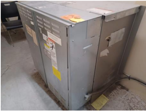
Photo 13: View of the hydraulic unit for the passenger elevator for the medical office on the second floor at 1105 E Kingston Road.
