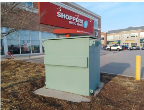
Photo 9: View of the transformer east of the Site building at 1105 D Kingston Road. Photograph taken facing north-east.
