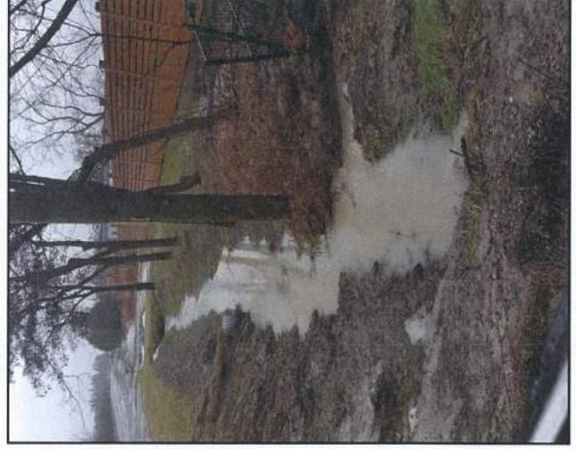
Photograph 32. Downgradient view of outlet of intermittent swale/drainage ditch into Old Brock Road ditch along subject property frontage, showing lack of sediment fencing/straw bales that have allowed surface water runoff, sediment runoff and pumped excavation water from 5321 Old Brock Road to be flushed downstream, underneath Old Brock Road and into part of the Glen Major Wetland Complex, a PSW, containing fish and fish habitat further downstream
