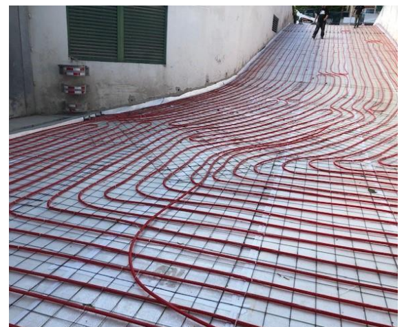
Glycol loop in underground parking ramp
