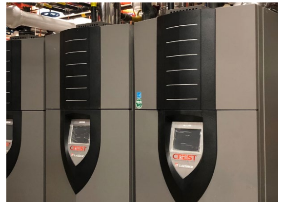
Boiler retrofit at Chestnut Hill Developments Recreation Complex
