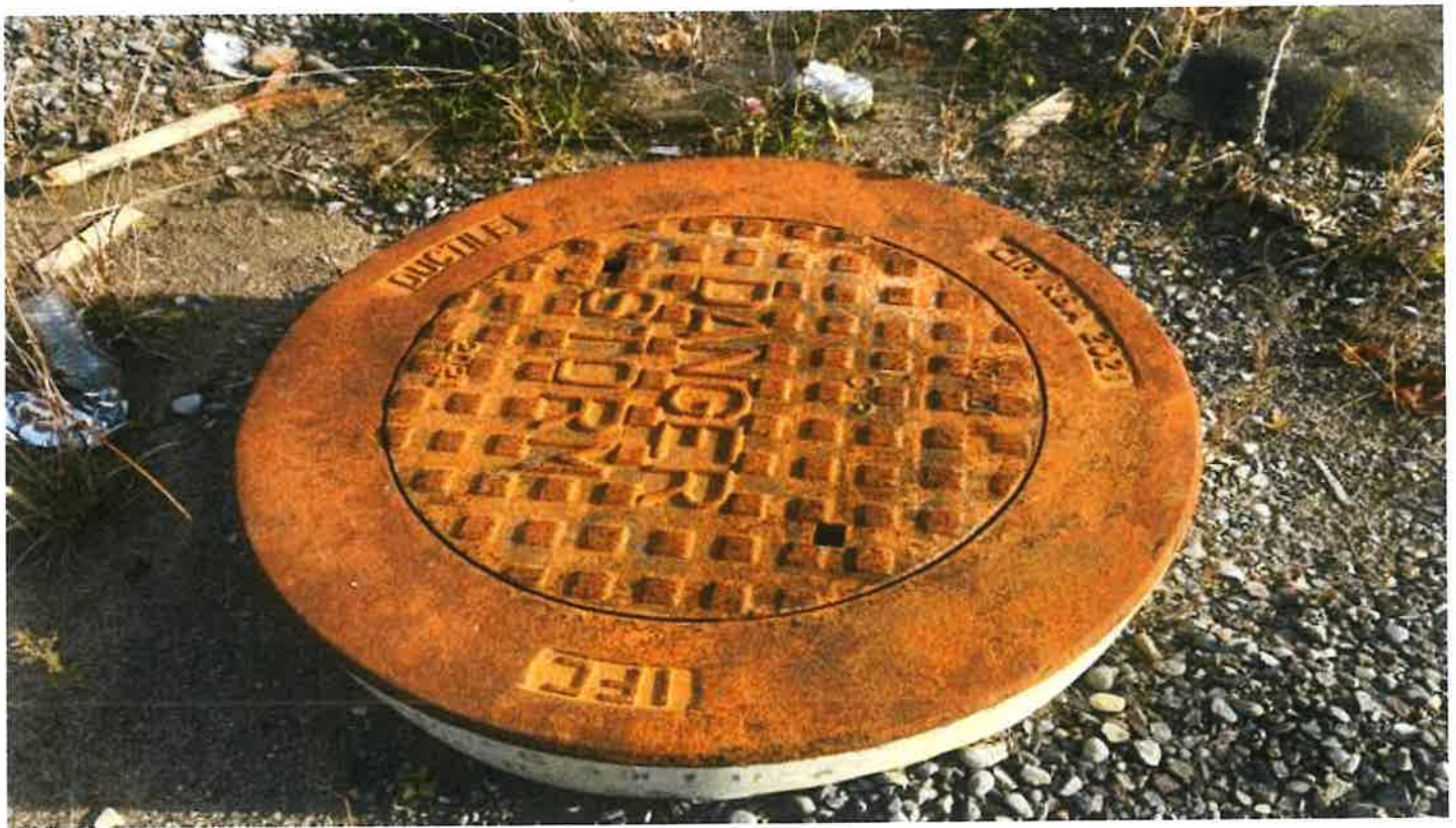
Close-up view of manhole in southeast portion of the subject site (looking north).
