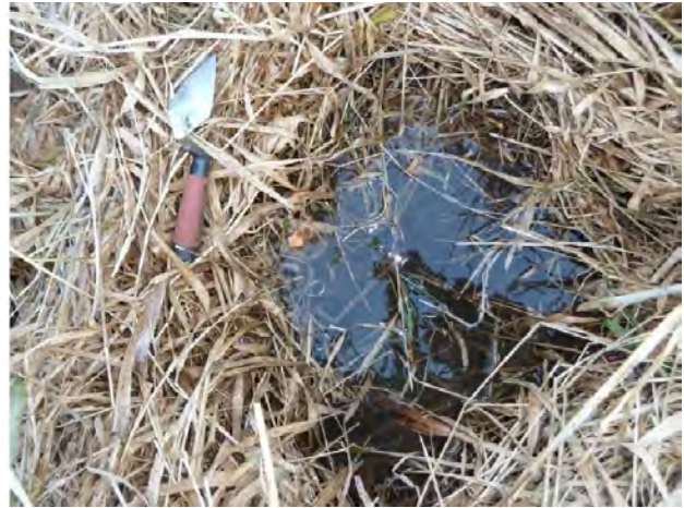
Photo 7: Close up of the bottom of the ditch pictured in Plate 6 showing wet conditions.
