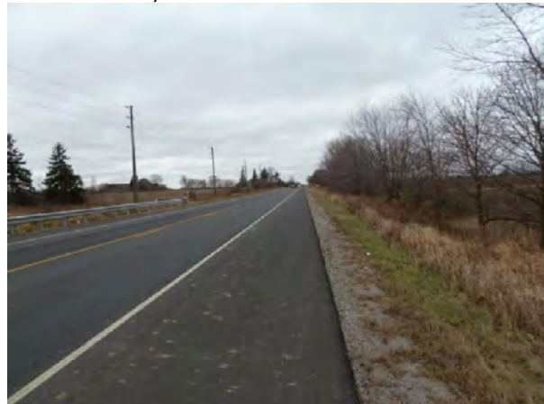
Photo 5: View southwest of the north side of Hwy 7 ROW with fill slope and ditch. Disturbed—no pot'l.
