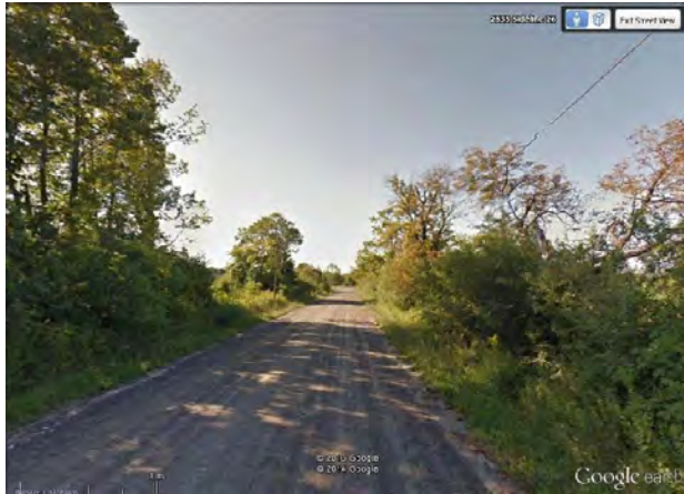
Photo 127: Survey Unit WM2-h—View SE along 26 Sideline. Disturbed ROW—no potential. Test pit survey conducted on both sides. Google Earth™.
