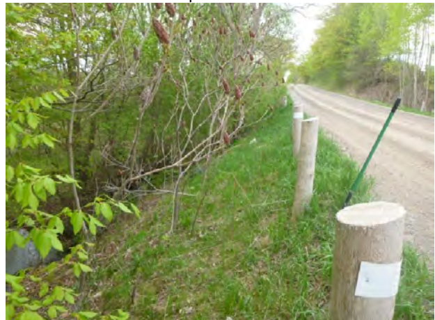
Photo 42: View south southwest. Steep fill slope east side of 16 Sideline. Disturbed—no potential
