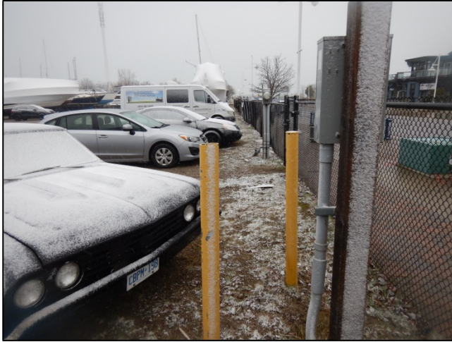
Photo 1: Evidence of underground hydro utilities along west side of parking area, facing southeast
