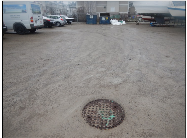
Photo 4: Underground water utilities in parking area, facing northwest
