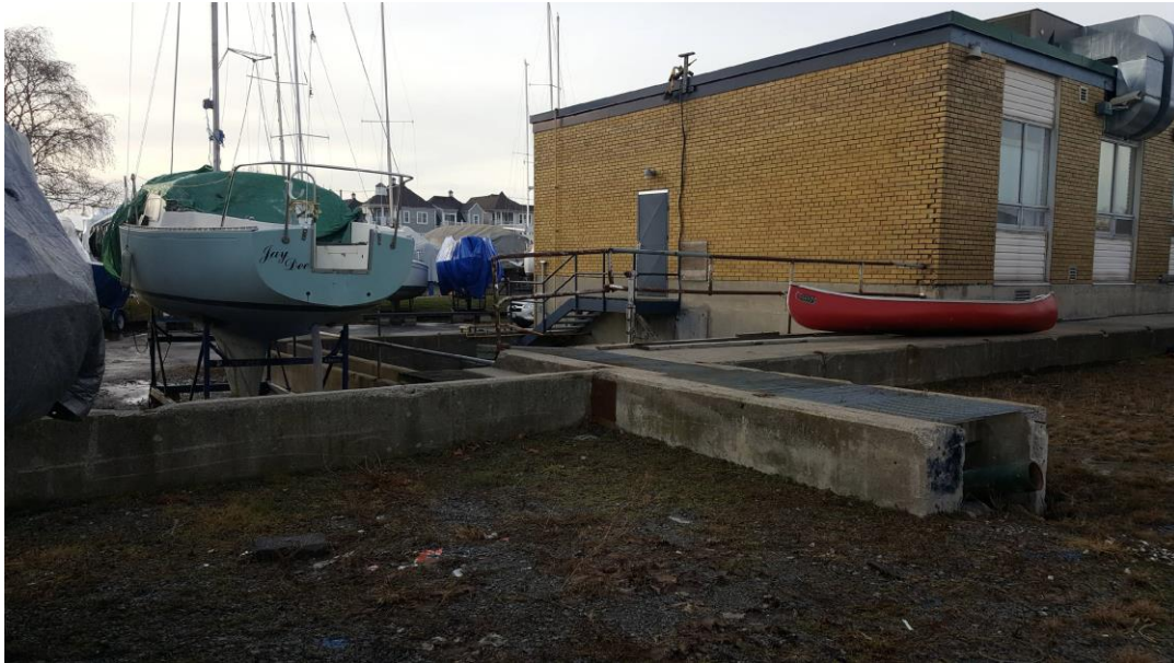
Photograph 5: View of concrete duct reaching concrete water holding pit located on the south side of the building.
