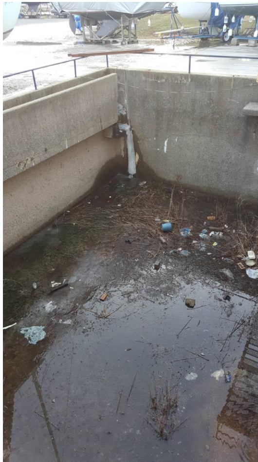
Photograph 6: View of concrete water holding pit located on the south side of the building.
