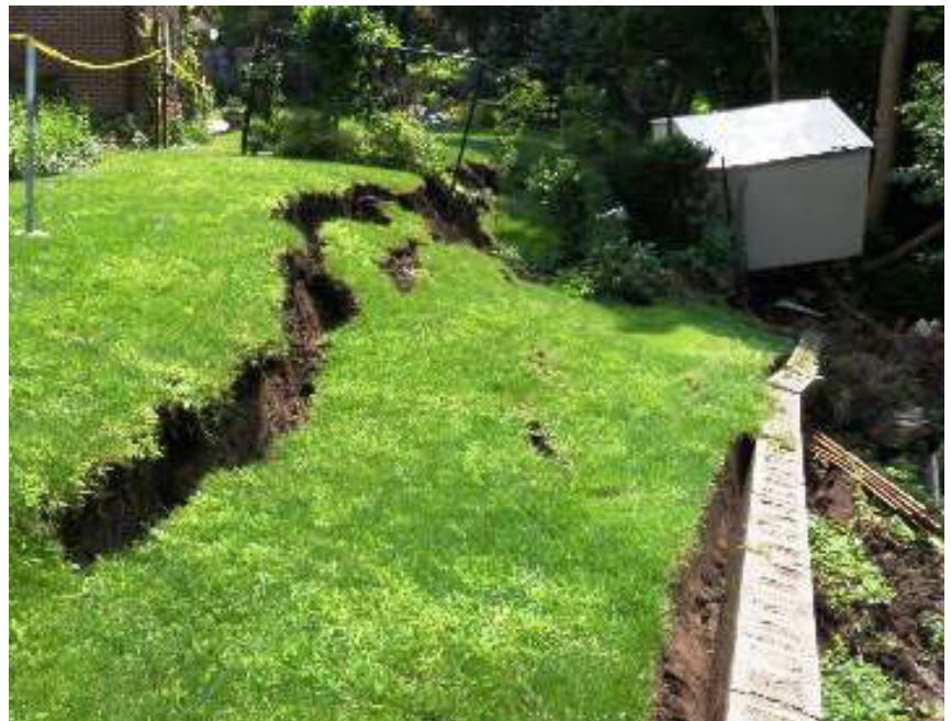
Illustration of a slope failure beside a home that is located in a natural hazard (Source: TRCA).
