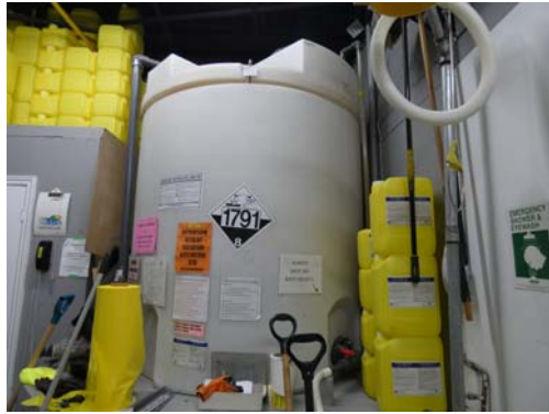
P37 - View of hypochlorite tank in rear room of units #637-639 Kingston Road
