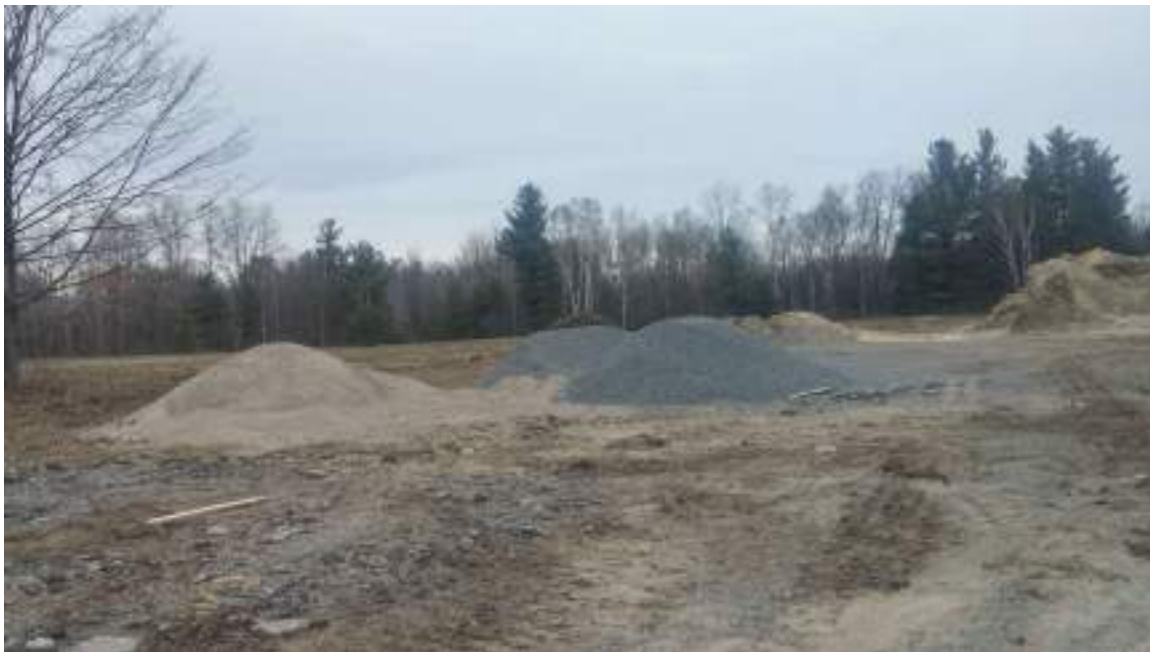
Photo 10 – View of stockpiles of gravel, sand and soil materials noted near the entrance of the West Portion of the Phase One Property (looking northeast).
