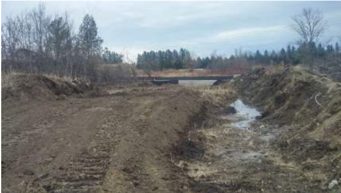
Photo 7 – View of the temporary entrance to the East Portion of the Phase One Property from a new public roadway (namely Dexshire Drive) (looking south).
