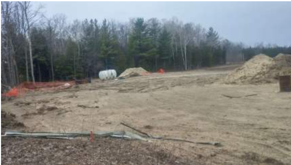
Photo 16 – View of soil stockpiles generated from two (2) excavated pits in the West Portion of the Site. A plastic storage tank was noted.
