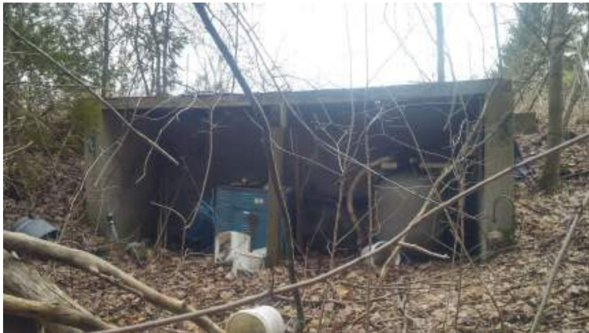
Photo 14 – View of a pool heater and filter storage area near the east edge of the West Portion of the Phase One Property (looking west)
