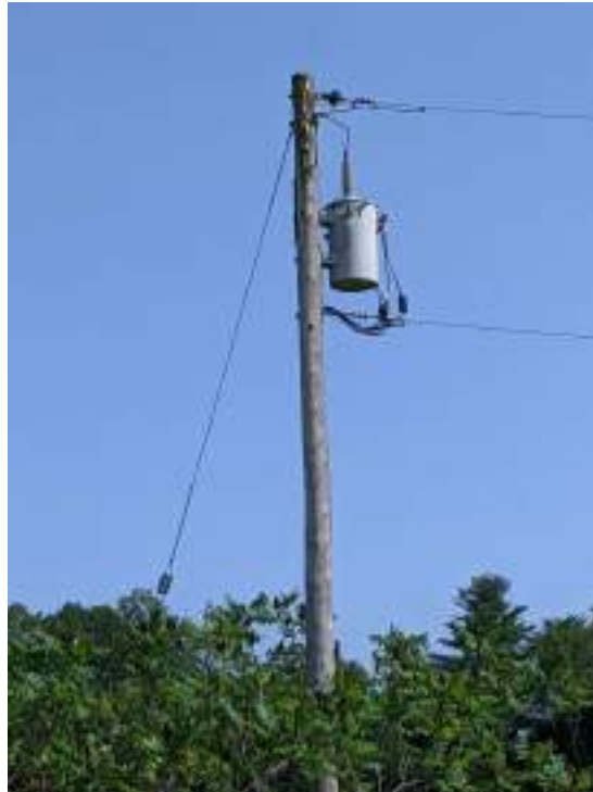
Site Photo 9. Transformer located on a telephone pole in the western portion of the Site. No spills, staining, discoloration or leaks observed.
