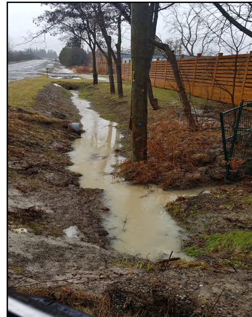
Photograph 32. Downgradient view of outlet of intermittent swale/drainage ditch into Old Brock Road ditch along subject property frontage, showing lack of sediment fencing/straw bales that have allowed surface water runoff, sediment runoff and pumped excavation water from 5321 Old Brock Road to be flushed downstream, underneath Old Brock Road and into part of the Glen Major Wetland Complex, a PSW, containing fish and fish habitat further downstream
