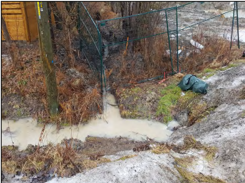
Photograph 31. Upgradient view of intermittent swale/drainage ditch (Oct 24 2020) showing lack of sediment fencing/straw bales with is allowing surface water runoff, sediment runoff and pumped excavation water to drain onto the subject property from 5321 Old Brock Road property to the south
