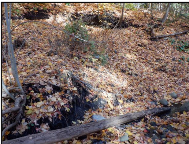
Figure 2-29: Erosion Site #20 – Toe Erosion Creating Risk to Private Property on Duncannon Drive.
