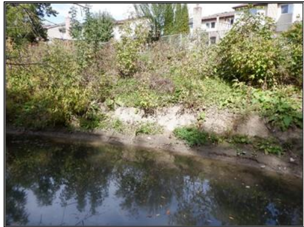
Figure 3-5: Unlined Channel with Sandy Banks Eroding at Meander less than 5m from Private Property.
