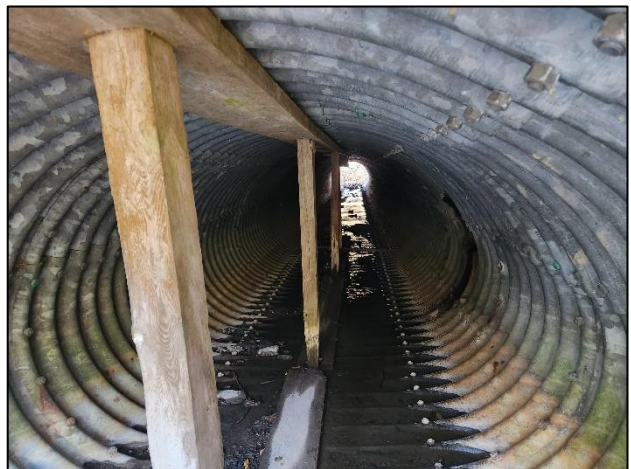
Figure 2-35: Erosion Site #22 – Wooden Support Posts Observed within the Lynn Heights Drive Culvert.
