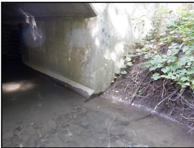
Figure 2-7: Erosion Site #5 – Minor Bank Erosion Downstream of the Glenanna Road Culvert Crossing.
