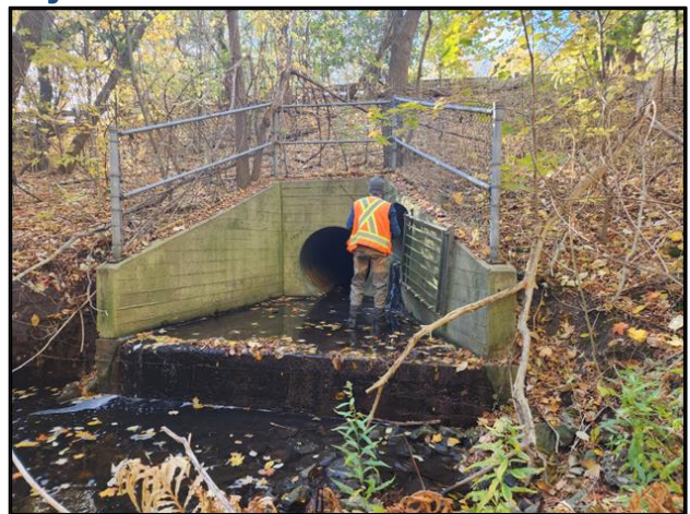
Figure 2-30: Erosion Site #21 – Significant Scouring Observed Downstream of Fairport Road Outfall.
