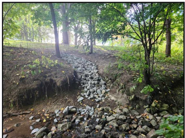
Figure 2-10: Failure of Rip-Rap Bank Treatment Intended to Prevent a Loss of Parkland due to Active Erosion Processes.
