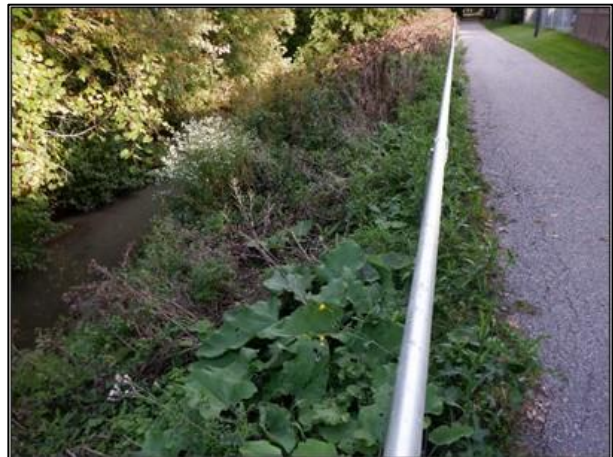
Figure 3-9: Looking Downstream from Trail Which is Within 2.0 m of Channel. Erosion Taking Place at the Toe of the Over Steepened Bank.
