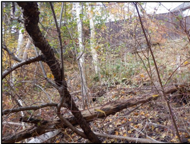
Figure 2-27: Erosion Site #17 – Toe Erosion Creating Risk to Private Property on Grafton Court.
