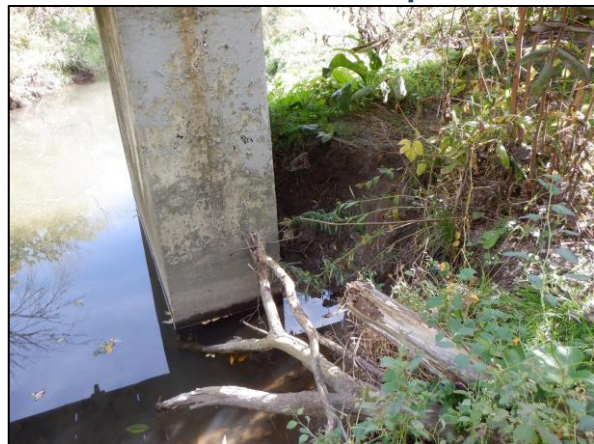
Figure 2-5: Erosion Site #4 – Scouring & Erosion around Bridge Footings
