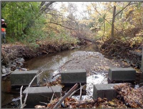
Figure 3-12: Sediment Accumulation Occurring Downstream of Energy Dissipation Blocks at the Dixie Road Culvert Causing Aggradation of the Bed and Active Channel Widening.
