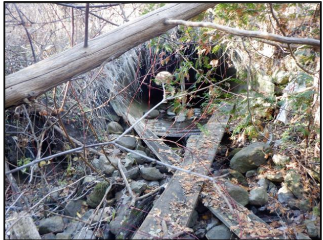
Figure 2-33: Erosion Site #22 – Observed Scouring Downstream of the Lynn Heights Drive Culvert.
