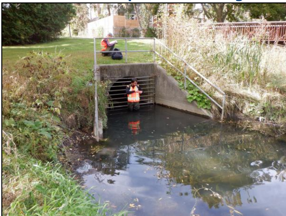
Figure 2-4: Erosion Site #3 – Outflanking of Concrete Wingwalls due to Erosion.
