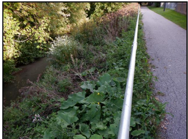
Figure 2-15: Erosion Site #10 – Bank Erosion Actively Encroaching Towards the Existing Multi-Use Trail
