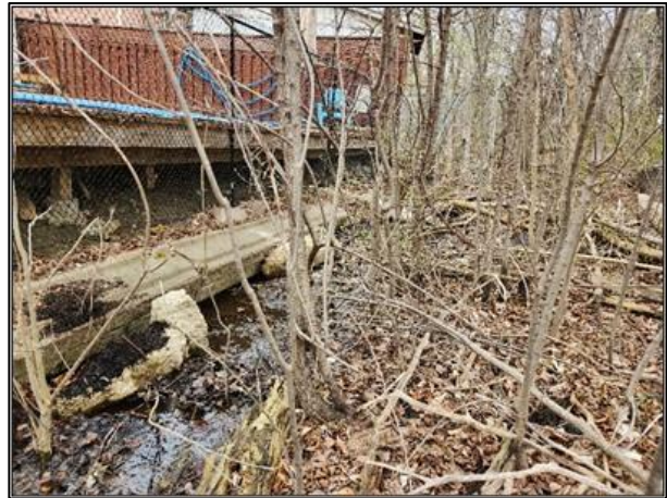
Figure 3-17: Looking Upstream near the Midpoint of the Reach. Note Encroachment of the Channel Towards Private Property.
