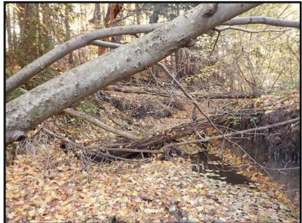
Figure 3-25: Erosion on the Outside of the Meander Bend Looking at the North Easterly Bank. Leaning Trees and Exposed Tree Roots Visible.
