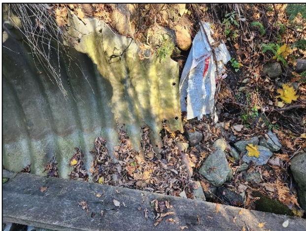
Figure 2-34: Erosion Site #22 – Observed Structural Degradation at the Culvert Outlet.
