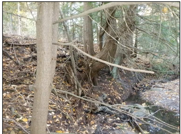
Figure 2-40: Erosion Site #24 – Actively Eroding Bank behind Duncannon Drive Properties.
