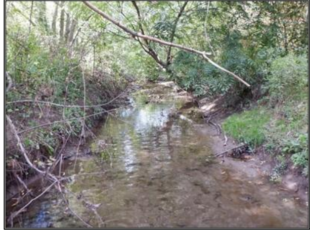
Figure 3-7: Looking Upstream at the Straight Channel where Bank Erosion Present Throughout the Reach can be Seen on Either Bank of the Channel
