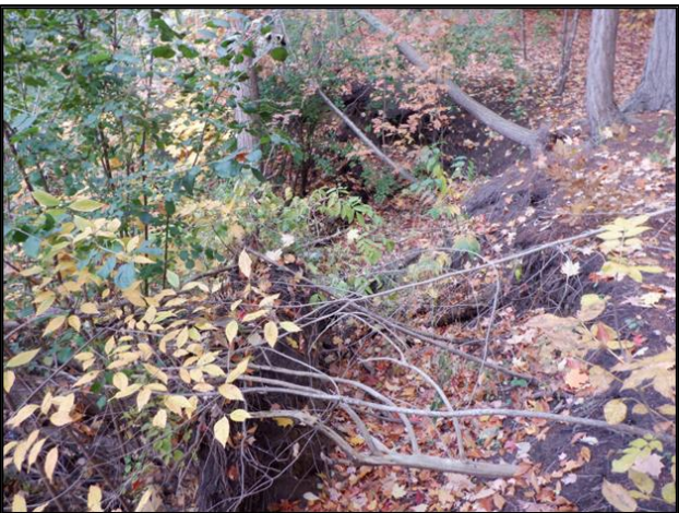
Figure 2-19: Erosion Site #12 – Mass Debris Jams Forcing Channel to Erode Eastward
