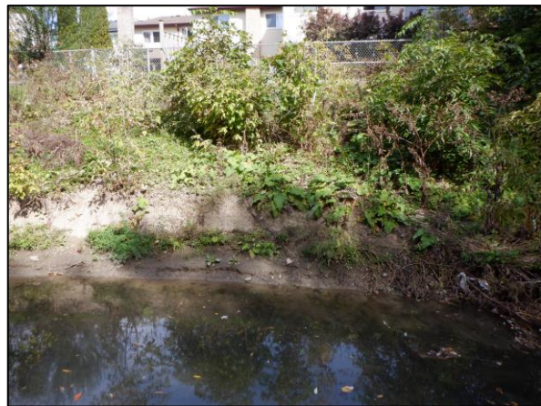
Figure 2-3: Erosion Site #2 – Bank Erosion Risk to Private Properties
