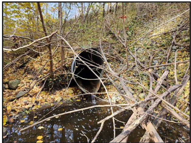
Figure 2-25: Erosion Site #16 – Undercutting of Deformed CSP Culvert
