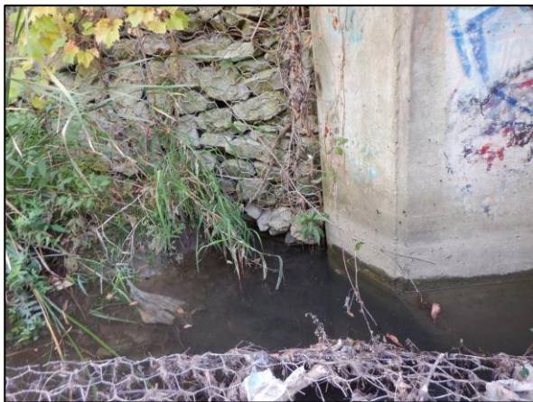
Figure 2-2: Erosion Site #1 – Undermined Gabion Baskets Upstream of Kingston Rd.
