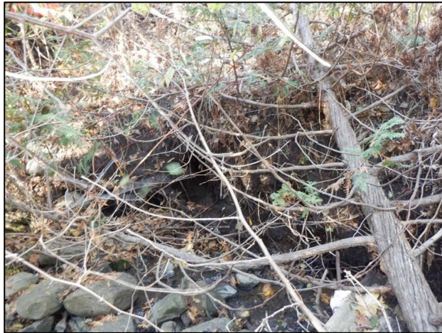
Figure 2-32: Erosion Site #22 – Debris Jam Downstream of the Lynn Heights Drive Culvert.
