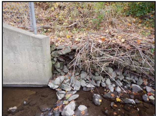
Figure 2-18: Erosion Site #11 – Observed Gabion Basket Failure
