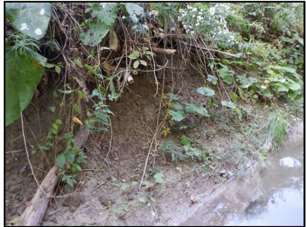
Figure 2-13: Erosion Site #10 – Major Erosion Scar Adjacent to a Multi-Use Trail System
