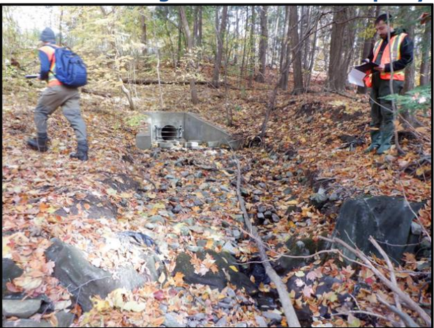
Figure 2-24: Erosion Site #15 – Eroding Outfall Channel
