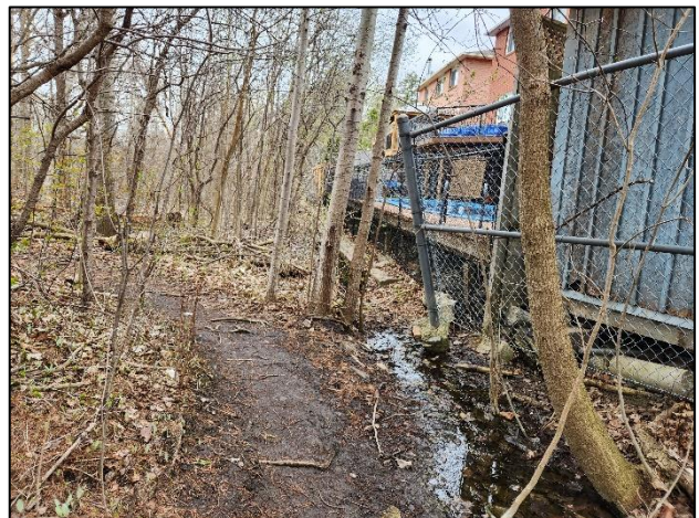
Figure 2-45: Erosion Site #25 – Encroachment of the Kitley Ravine Drainage Ditch towards Private Property.
