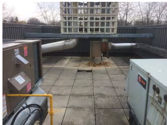
Photo 90 Rainfall Monitor Location
