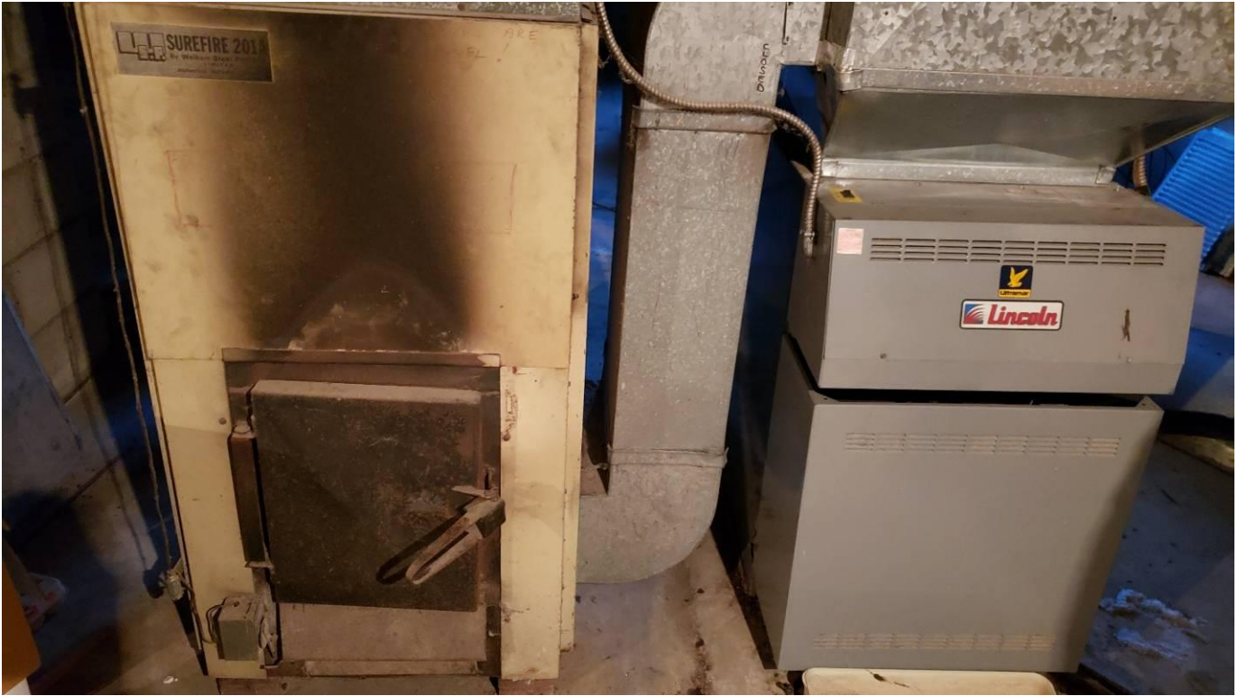
Photograph 7: In the basement of the house on subject property, showing the natural gas furnace.
