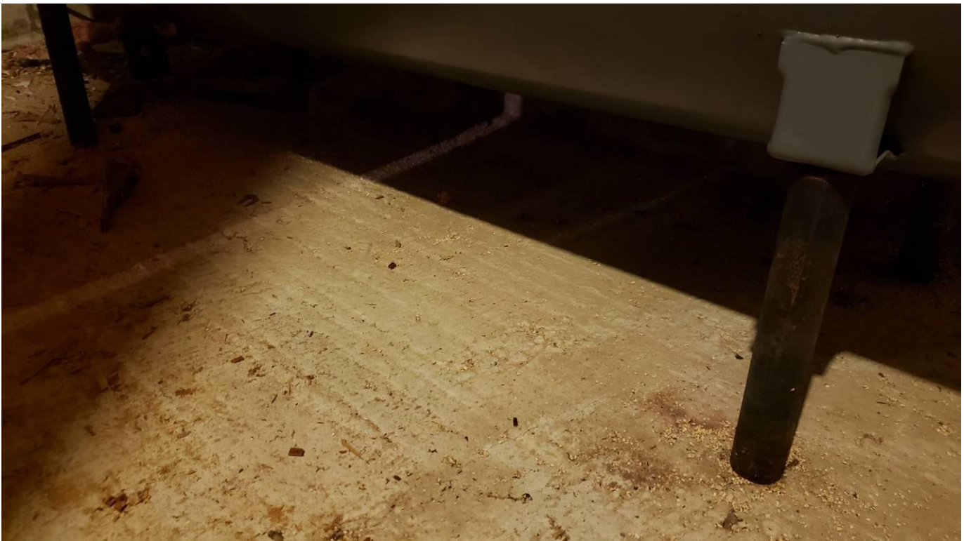
Photograph 8: View of the concrete slab in basement directly below the location of the empty oil fuel tank.
